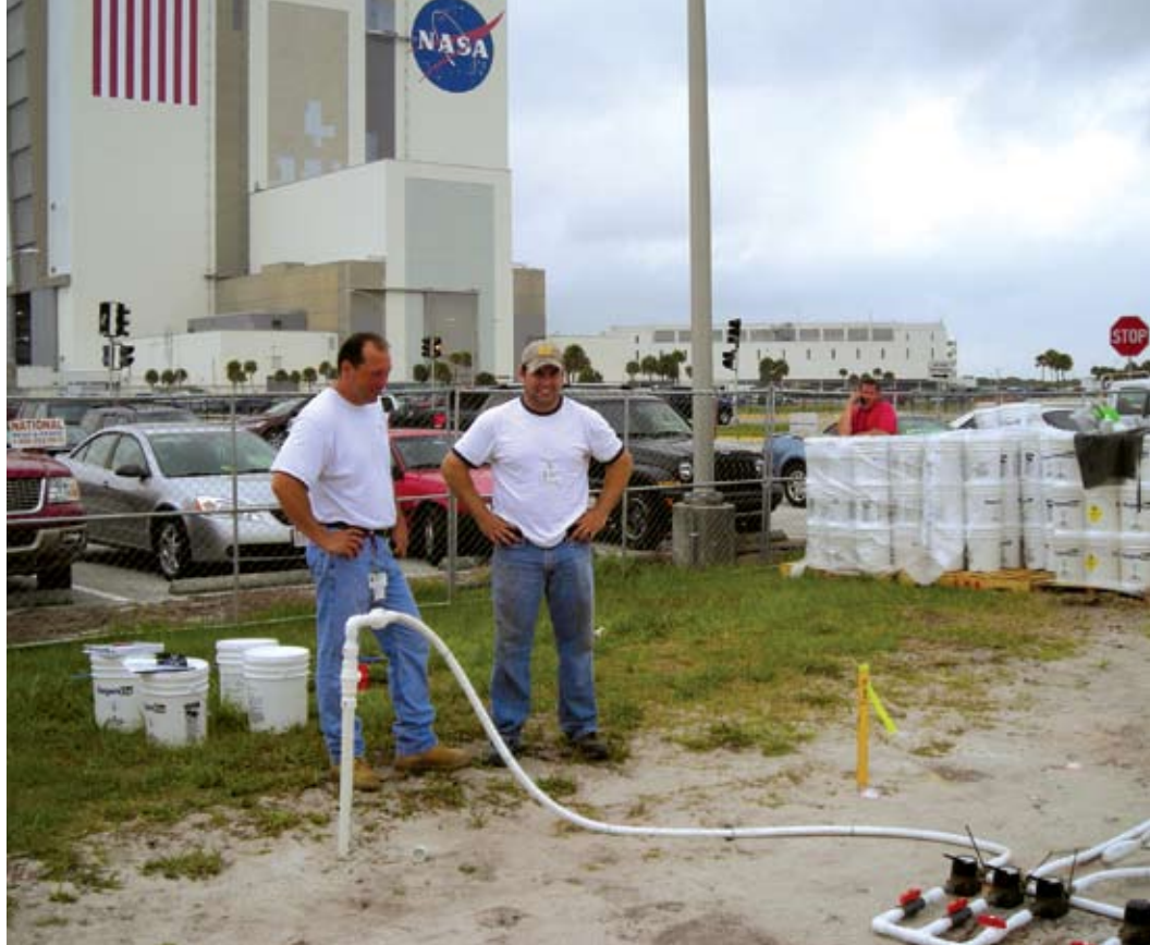
A multi-catalytic formula was injected into the injection points to treat the contaminated soil and groundwater in place.
